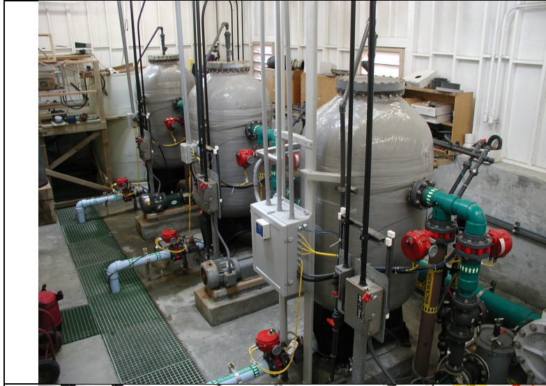
Figure D6: Seawater Intake Pumping and Filtration Plant Facility
